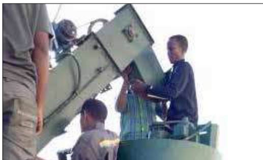
Starting the installation of the shredding, crushing and mixing agricultural residue machine
